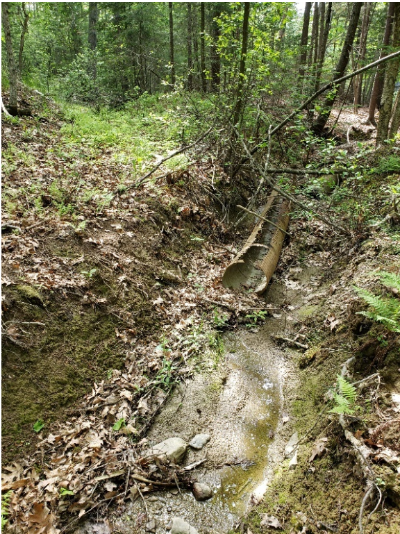
Photo 7: Broken culvert observed in sitting in the channel of Stream 5.
